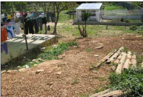
The present failing drain field at VS 1
